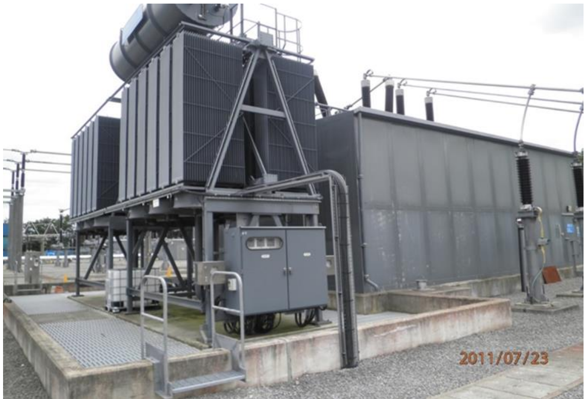
Image 4.5 Typical (large 400kV) power transformer
