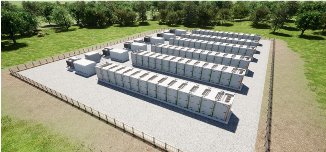
Image 4.7 Typical BESS Units
