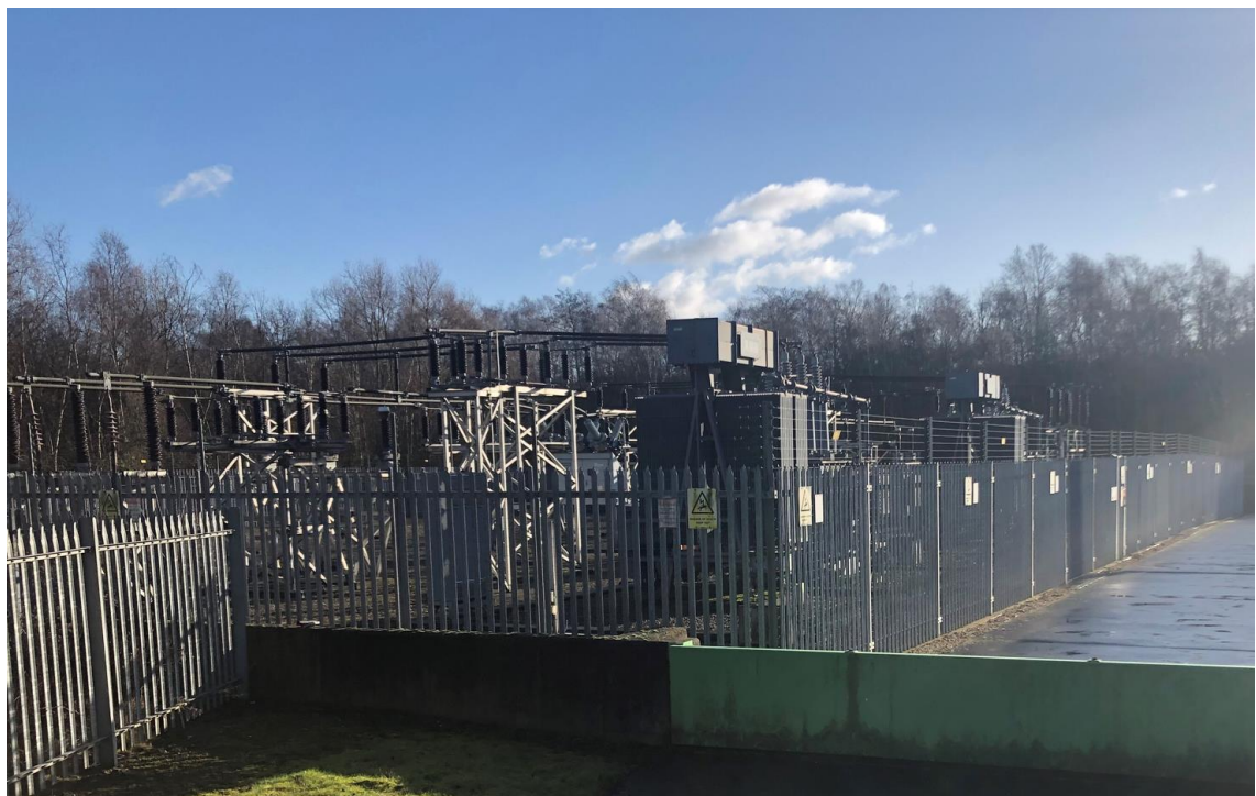
Image 4.6 Typical 132kV Substation Compound
